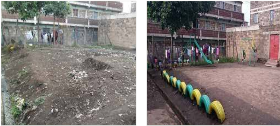
Transformation of a dumping space into a playground: before (left) & after (right)
